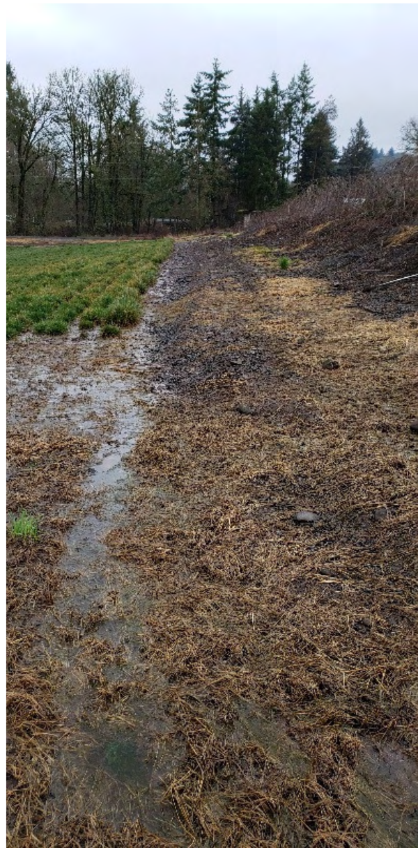
Photo 6: View of groundwater seeping along P1 boundary on January 6, 2020, facing north.
