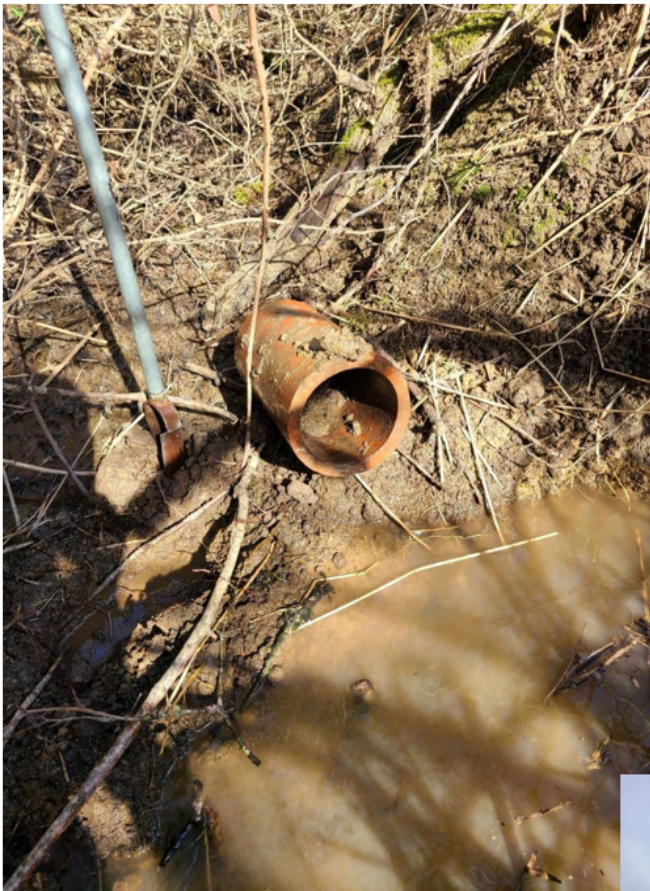
Photo 25: View of ceramic tile removed when digging up secondary tile outfall.
