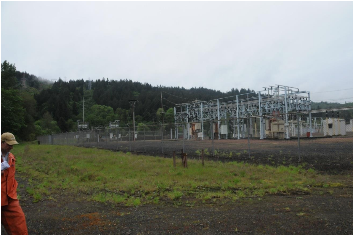
Sub Area 2, existing PGE substation. Taken 4/22/2016
