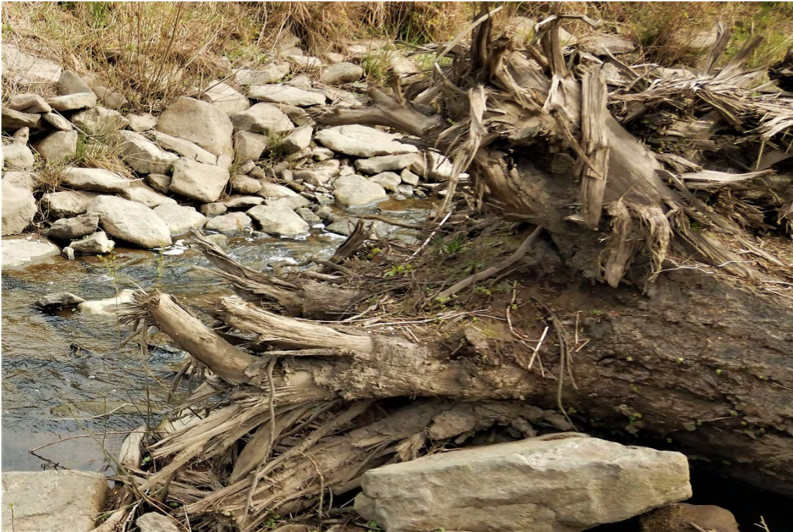
Figure 2-2. Typical Log Structure Installed and Retained Downstream of the Remnant Pond Outlet
