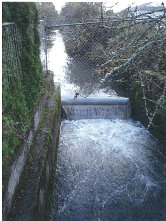
Figure 3. A weir upstream from Madras Road and the project area on Waln Creek. This structure limits the ranges of flows in the project reach as well as the influx of sediment.
