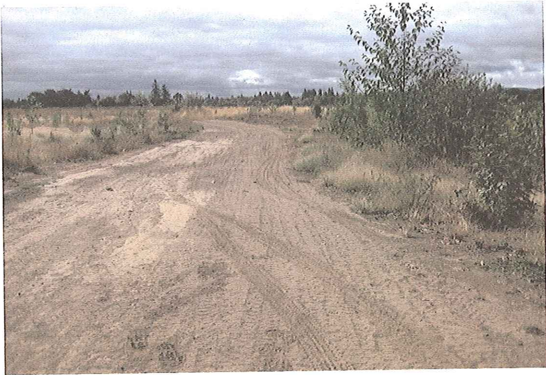
Photo Point 3 SE: Photo displays the un-improved access road which crosses the constructed swale.
