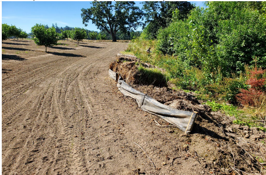
Photo 3. TESC at sediment encroachment location.
