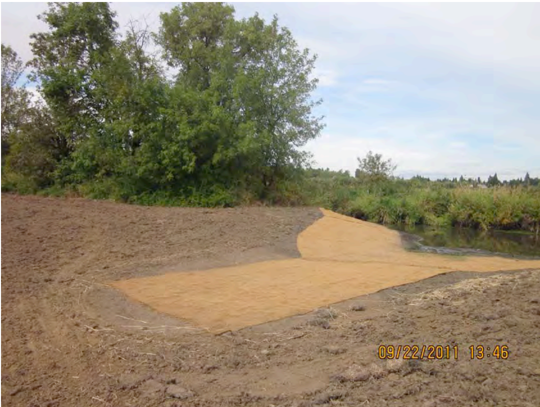
Photo 6 - North inlet into mitigation site regraded from filled Jackson Slough facing northwest.
