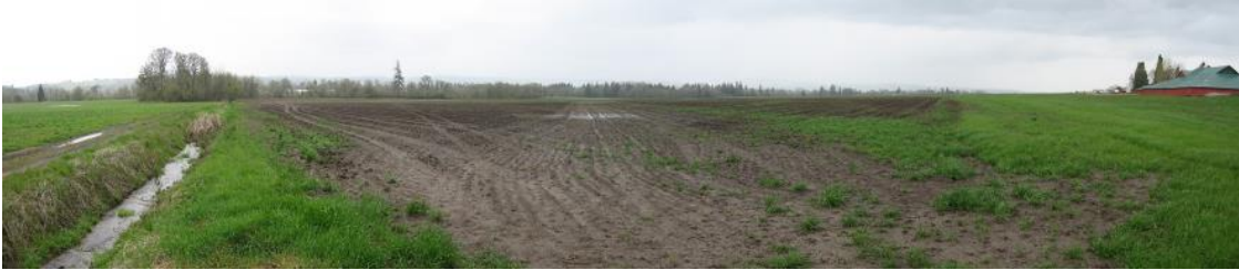
3/2014- Northern portion of east field after clearing of ground and before construction. Photo taken from NE corner.
